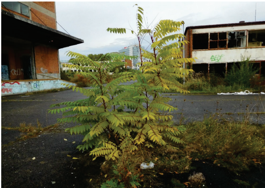
Fig. 5. Former logistic center of the American Forces at Frankfurt-Rödelheim. Ailanthus altissima growing in pavement cracks (Photo: G. Kasperek, 17.09.2016).
